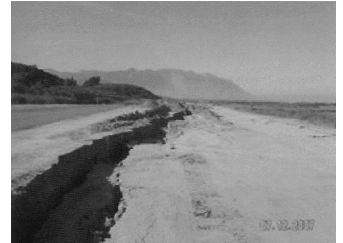
Crack and settlement (Athens-Thessaloniki highway)
