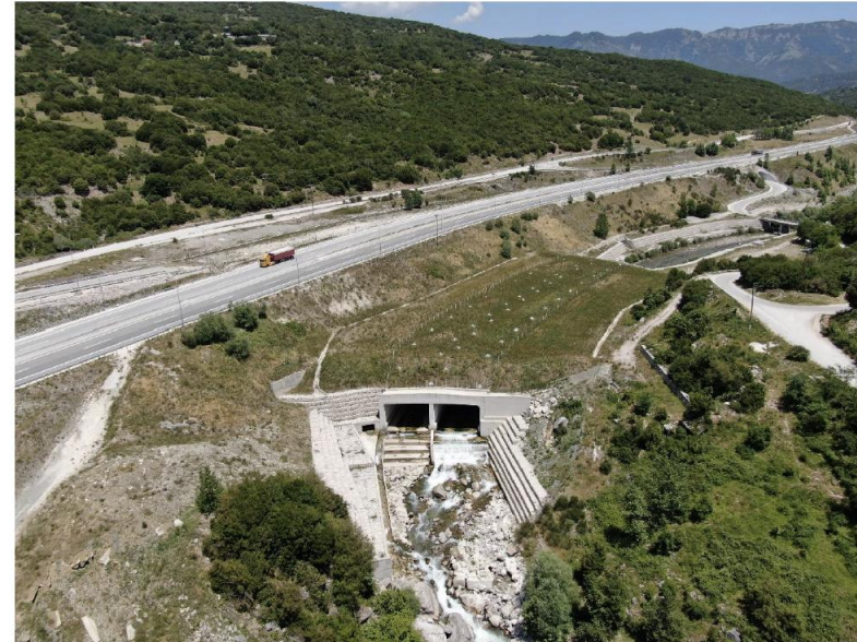
Twin tunnel of Metsovitikos River with berm above it stabilizing one landslide to the north (left side) and to the south (right side). Picture taken by drone from downstream of the river.
