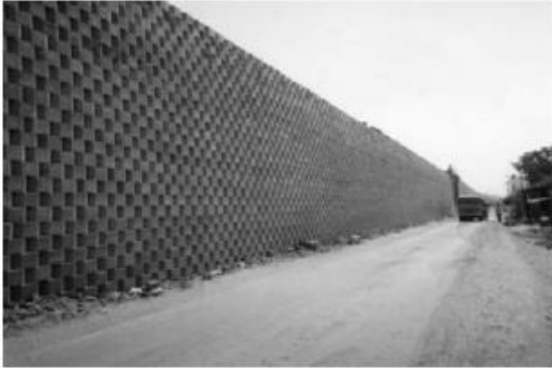
Figure 10.2. Oblique frontal view of geogrid reinforced segmental retaining wall at NH-5, Bypass near Kanpur [4]
