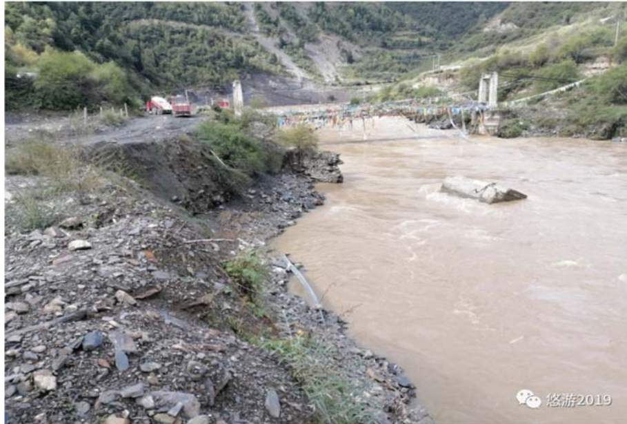
Figure 3.60 Riverbank morphology in the damaged section of retaining wall.
