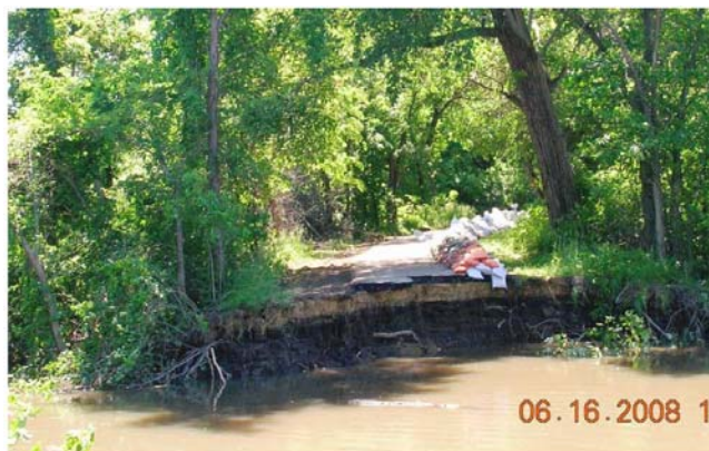
Figure 3.18 View looking to the southeast over the Birdland Levee breach (16 June 2008).
