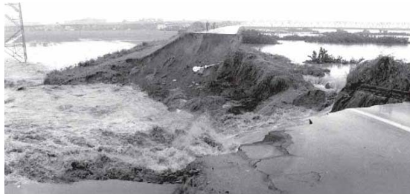
Just after breach
