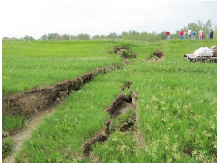
Figure 3.13 The initial distress in the levee L-575.
