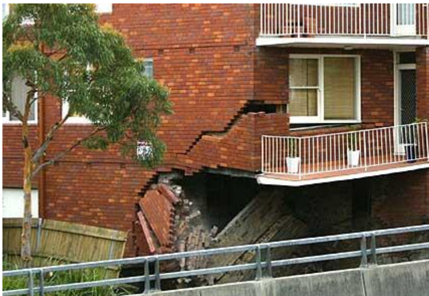
Figure 1: Building damage resulting from the collapse at the intersection of the Marden Street ventilation tunnel and the Pacific Highway Exit Ramp, Lane Cove Tunnel Project, Sydney, 2 November 2005
