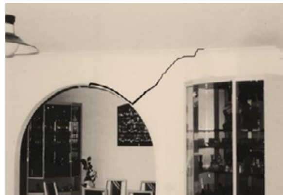
Figure 10: Cracking in wall
