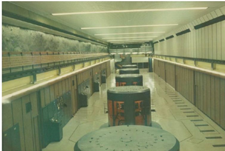
Figure 2: The completed Poatina underground power station
