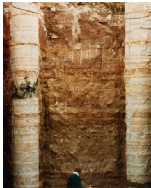
Figure 1: Piles excavated to examine construction defects
