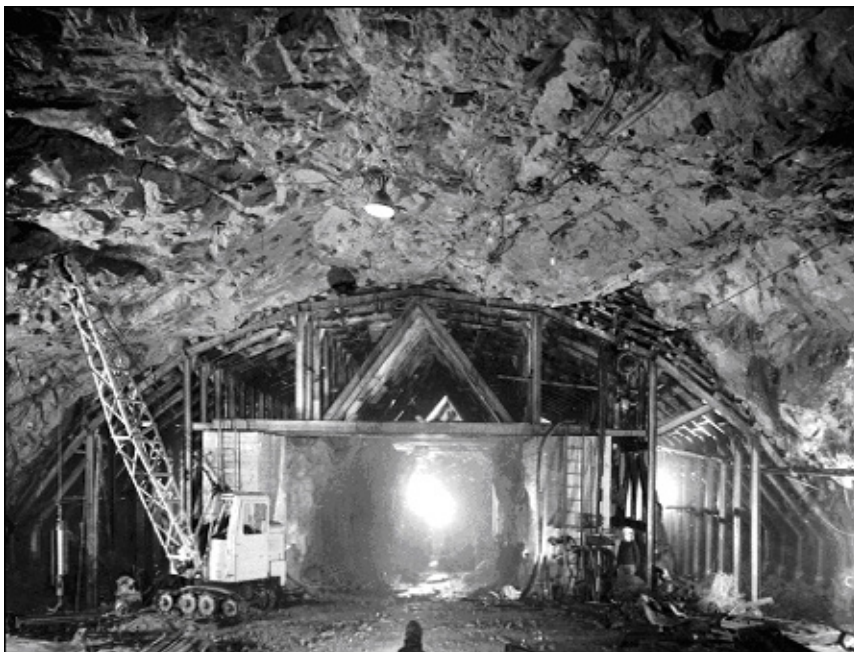
Figure 9: Tumut 1 power station during excavation of the roof section of the machine hall cavern (Endersbee, 1999)
