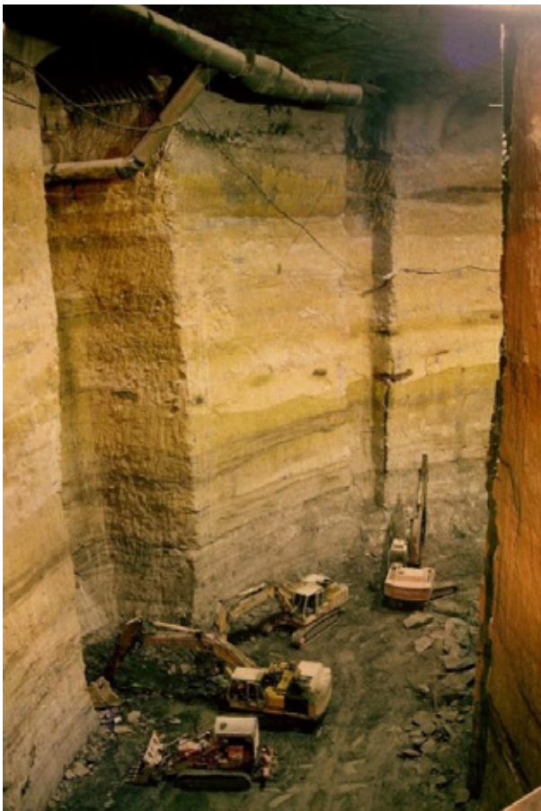
Photograph 4: Slots cut in side of cavern for the lifts and ventilation risers
