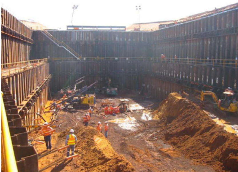
Construction of car-dumper infrastructure CD4 in Port Hedland with significant anchored sheet pile walls
