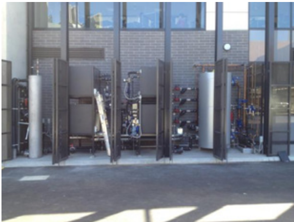
Figure 5: Heat pumps and other surface components at EBSS
