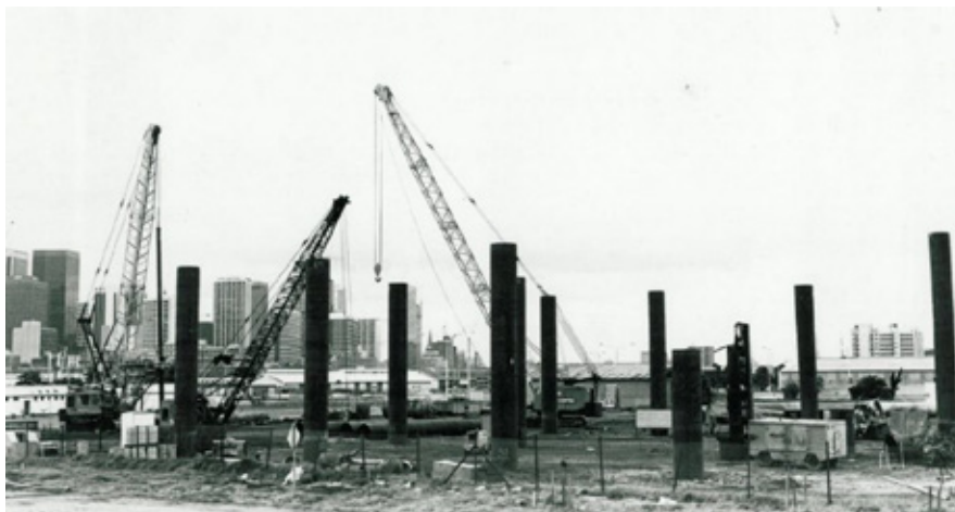
Westgate Freeway – South Melbourne
