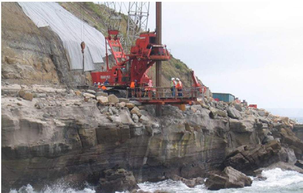
Figure 5: Drilling of a bored pile for Pier C in GD3 Photo courtesy of RTA
