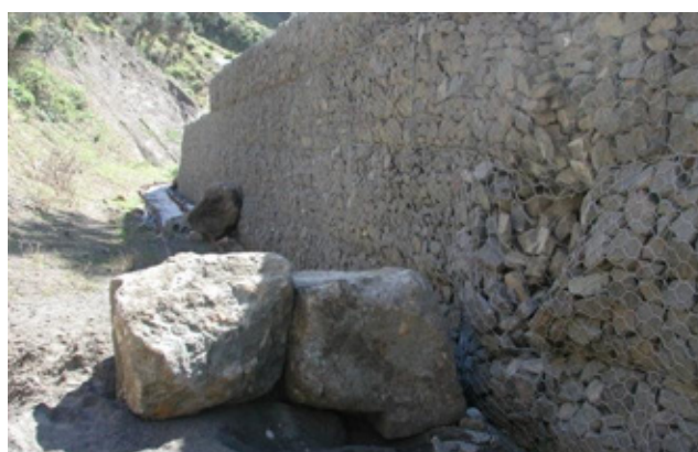
Figure 6: Debris termination bund and catch ditch in GD4 Photo courtesy of RTA
