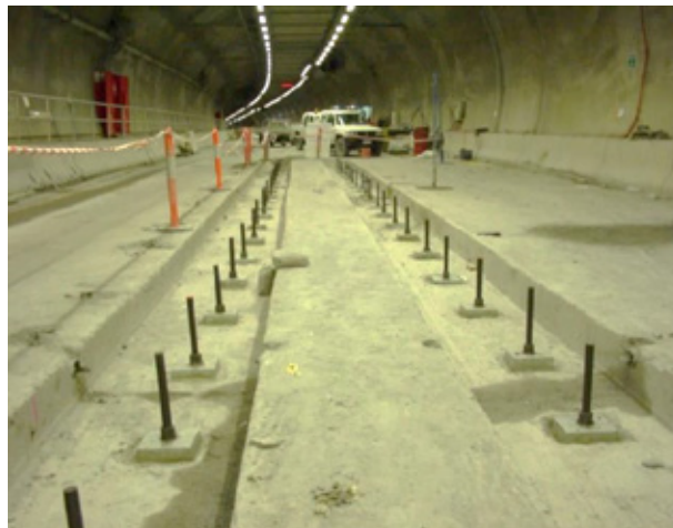
Photograph 3: Twin rows of anchors installed either side of the central invert joint in slabs which had not cracked
