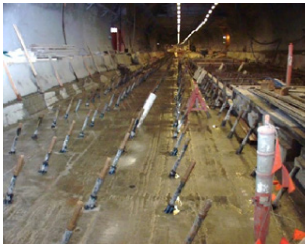
Photograph 2: VSL stressbar anchors installed after upper part of slabs removed; after stressing that upper part was reinstated with reinforced concrete
