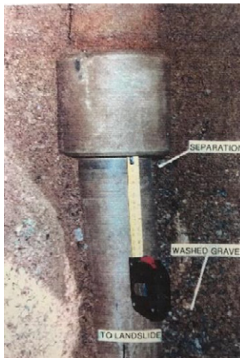
Figure 4: Joint 1 – as exposed
