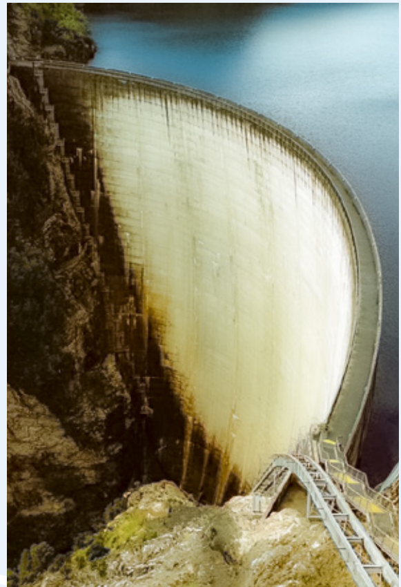
The double curvature concrete arch Gordon River dam in Tasmania, completed in 1974. Photograph courtesy Stephen Fityus
