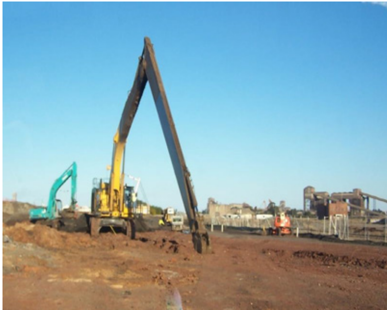
Long reach excavator constructing the upper part of the slurry cut-off wall to depths of up to 49m at the former BHP steel site, during an AGS Newcastle Chapter excursion in 2003
