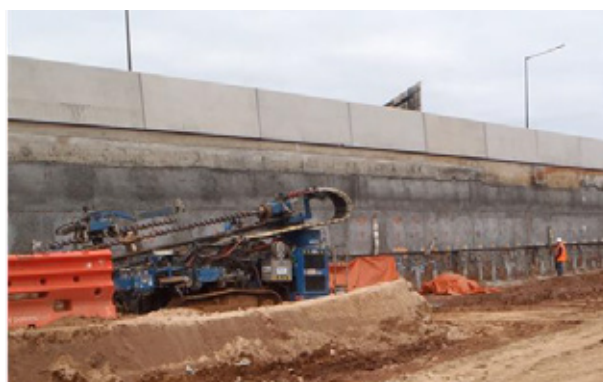
Figure 4: Light-weight soil nail/sprayed concrete retaining walls up to 10m high on the Torrens to Torrens Project
