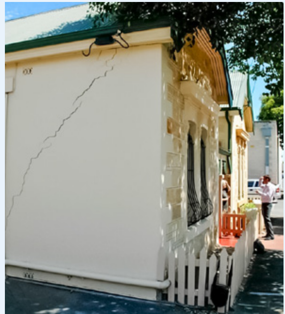
Cracked house in Adelaide Photograph courtesy FMG Engineering
