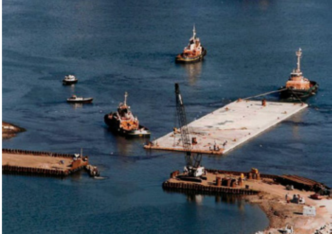
Figure 5: An IMT Unit being towed out of the Cofferdam at Port Kembla (courtesy of Ms Margaret Rush)
