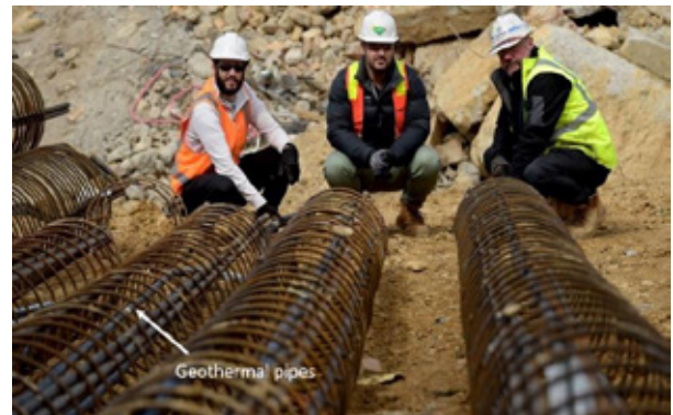
Figure 6: HDPE geothermal pipes fixed in pile cages for the Melbourne Connect building
