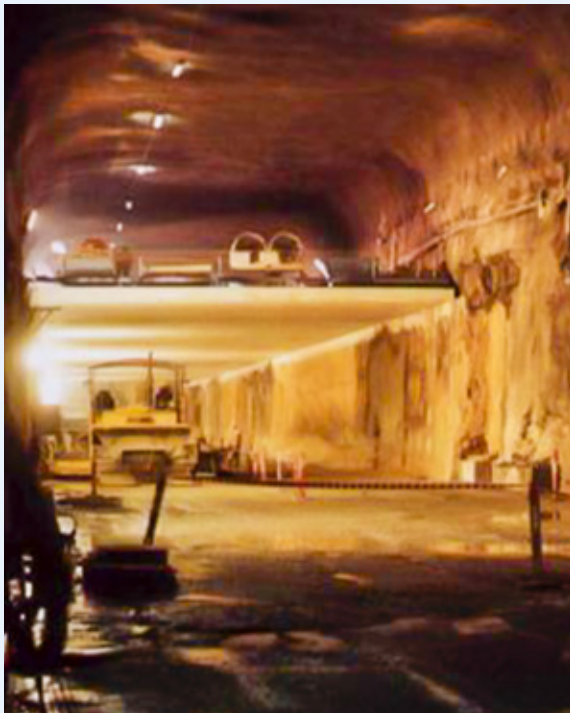
Eastern Distributor Tunnel, Sydney, opened in 1999 Photograph from front cover of Australian Geomechanics June 1999
