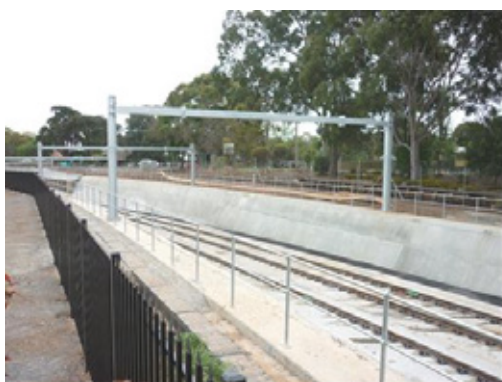
Figure 3: Six metre high revetment in unsaturated clay on the eastern approach to the Goodwood rail underpass
