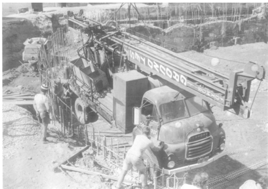
Ground Test drilling rig being lowered into the excavation at the Newcastle City Council 'Roundhouse' Building in 1972
