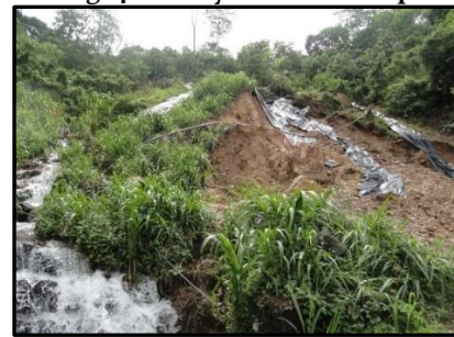
Fig. 5 Stream beside the landslide
