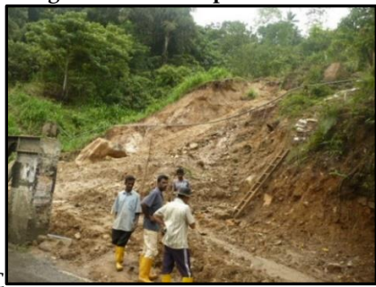
Fig. 3 Failure after toe excavation
