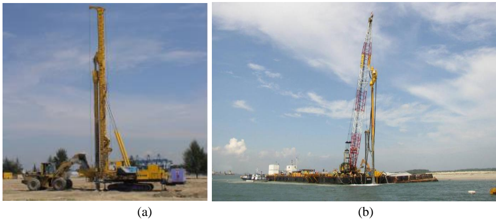
Figure 26. Vibro replacement system (a) dry bottom feed system and (b) a free hanging installation system for offshore works
