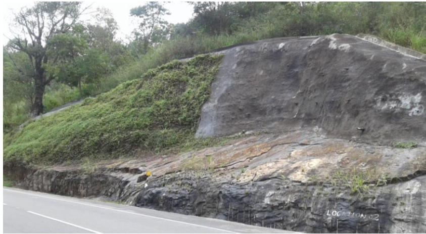
Figure 2.33 : Mitigation Measures with Soil Nailing, Drains and Facing with Shotcreting and Vegetation
