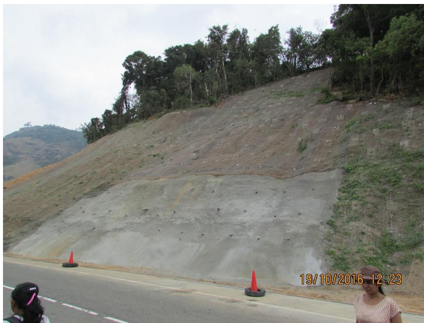
Figure 2.34 : Mitigation Measures with Soil Nailing, Drains and Facing with Individual Pillows Connected by High Tensile Wire Mesh, and Vegetation
