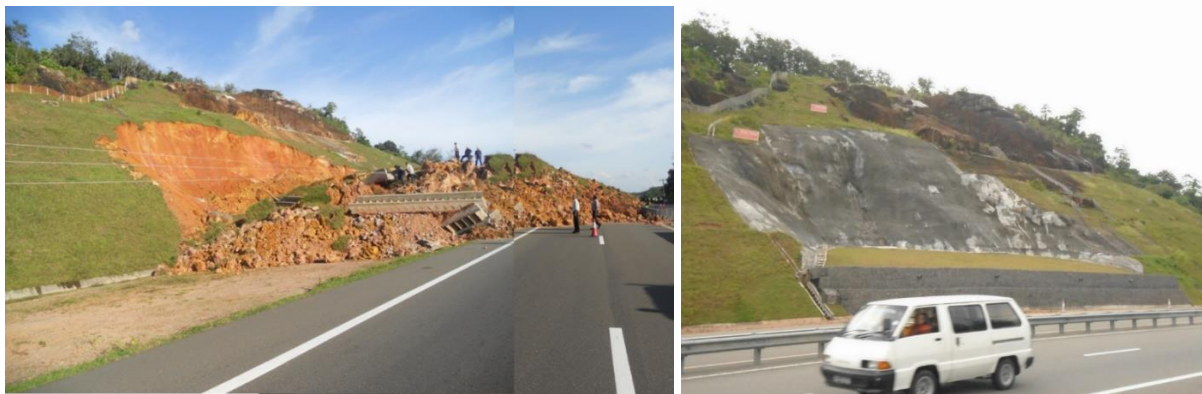
(b) After Failure (a) After Rectification Figure 2.31 : Failure at Welipenna on Southern Expressway (Idirimanna, 2016)
